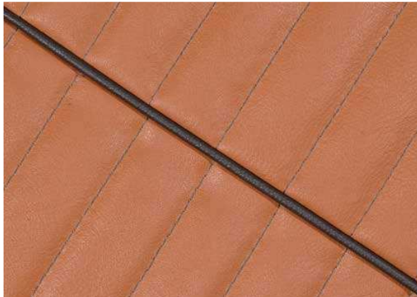
Tan / Black piping
